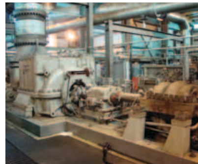
Process air compressor, compressor train.
